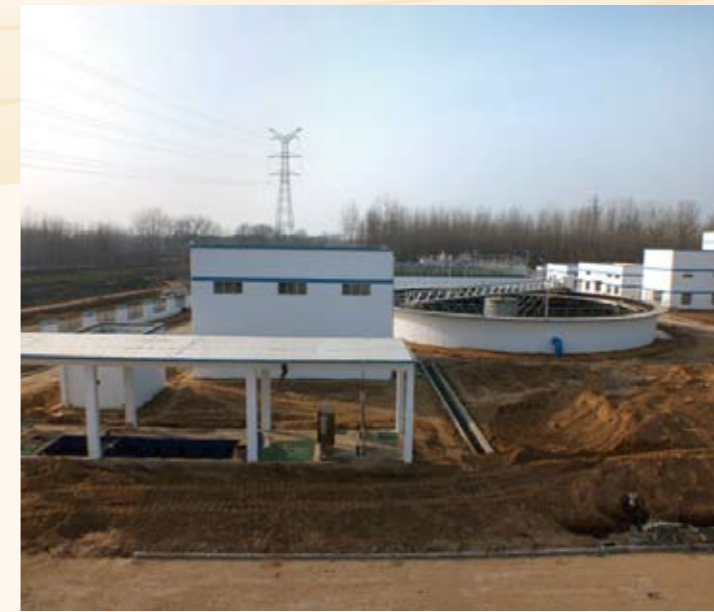
江苏宿迁城北污水处理厂一期工程 Jiangsu Suqian Chengbei Wastewater Treatment Plant Project (Phase I)
