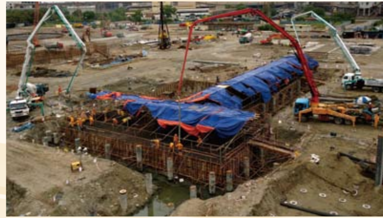
马来西亚Prai CCGT电厂土建施工项目 Onshore Civil Work Project of Malaysia Prai CCGT Power Plant
